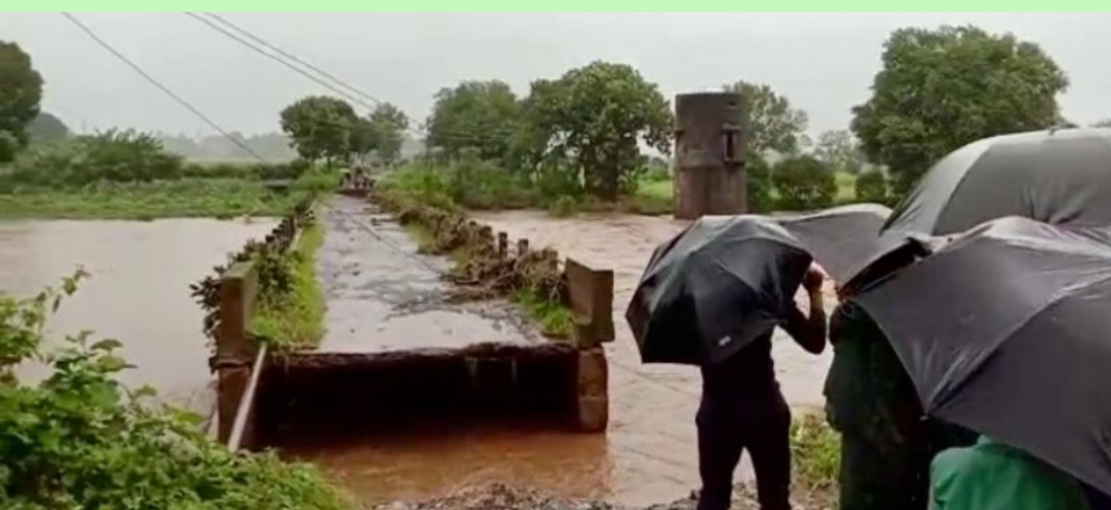
Bridge in Hunswad village of Haliyal that suffered serious damage during the floods
